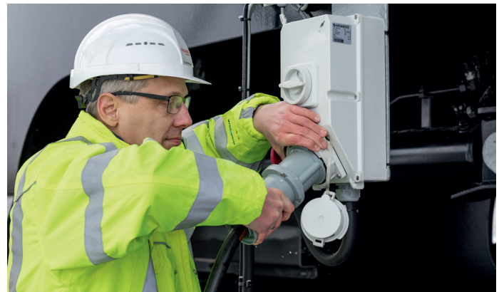
Charging of the batteries is also possible when the crane is connected to an auxiliary power source of min. 400V/63A
